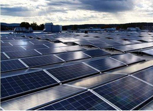
Figure 4-6 Roof Mounted Solar Panels Angled East-West in Adjacent Rows
